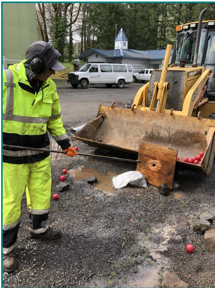
Paul Walker demonstrates the power of the high pressure hydro excavation wand by cutting through a piece of plywood.
