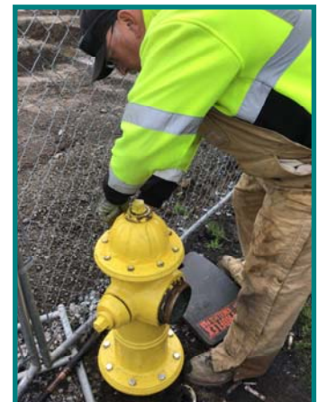
New Fire Hydrant
