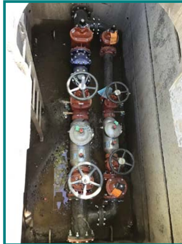
New Meter & Bypass
