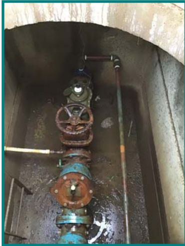
Old Meter & Bypass
