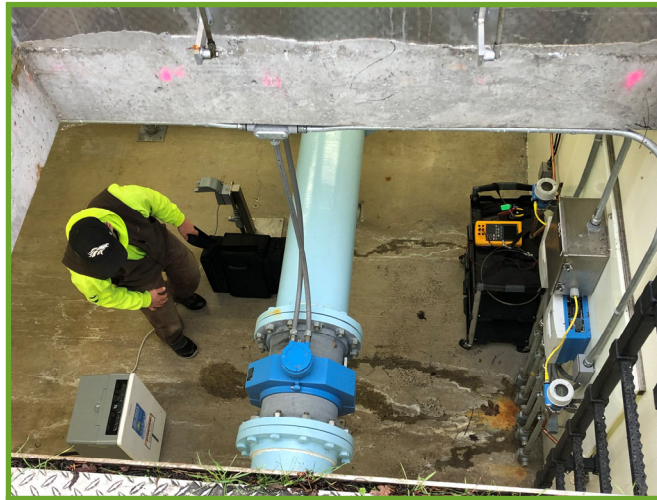
Measuring flow with ultrasonic flowmeter
