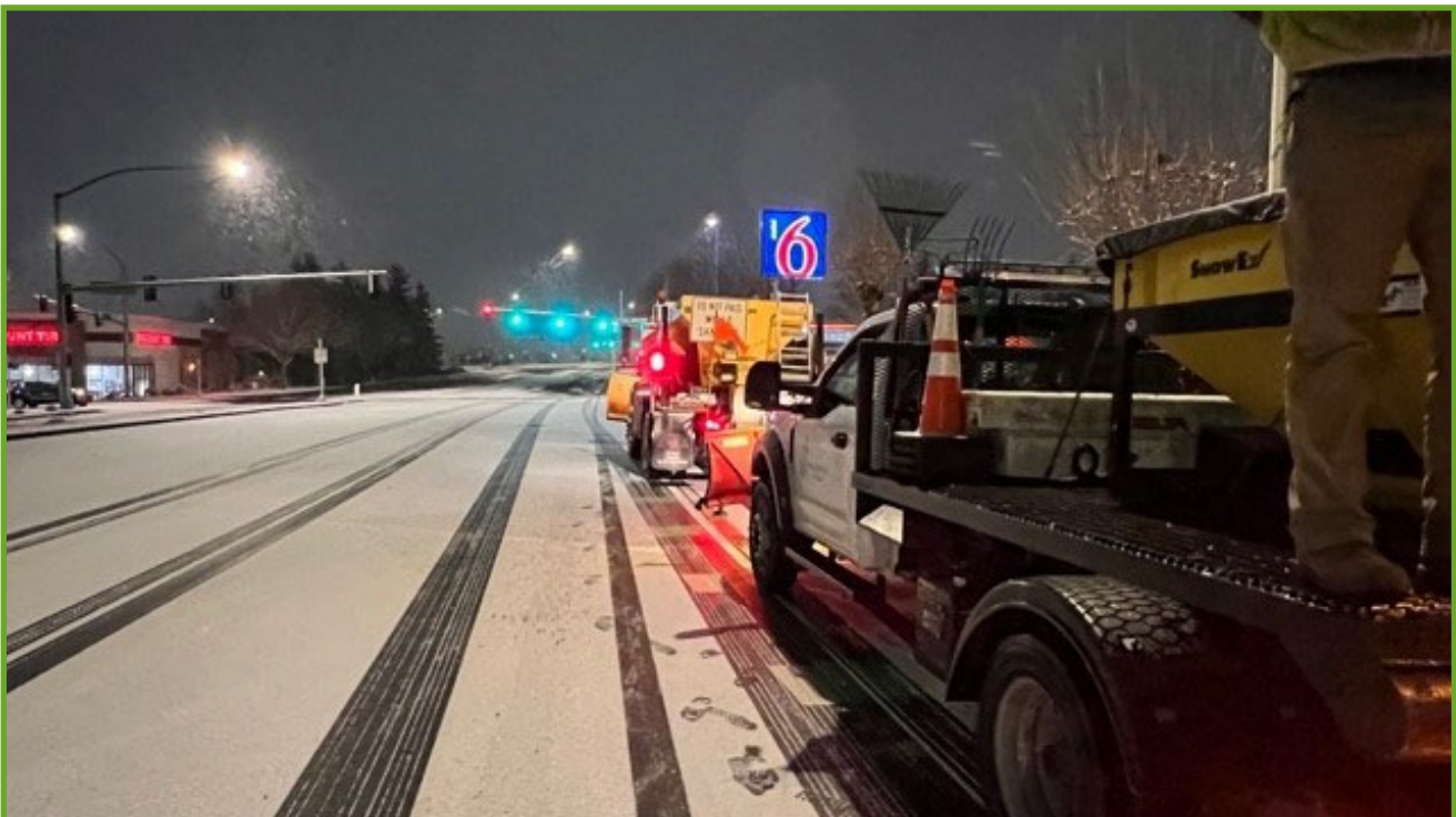
Sanding equipment on Elligsen Road
