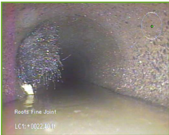
Root intrusion into sewer pipe
