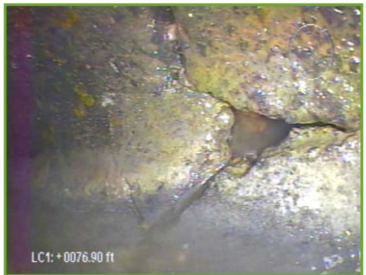
Crack on side of sewer pipe
