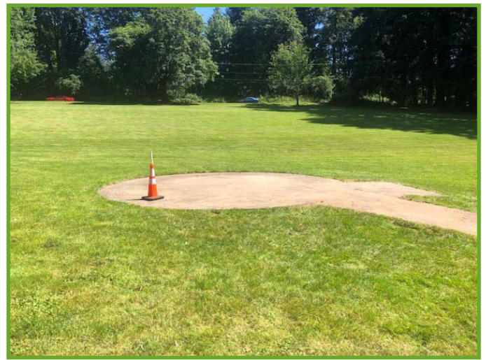
After complete removal and cleaning of the area where the Gazebo once stood
