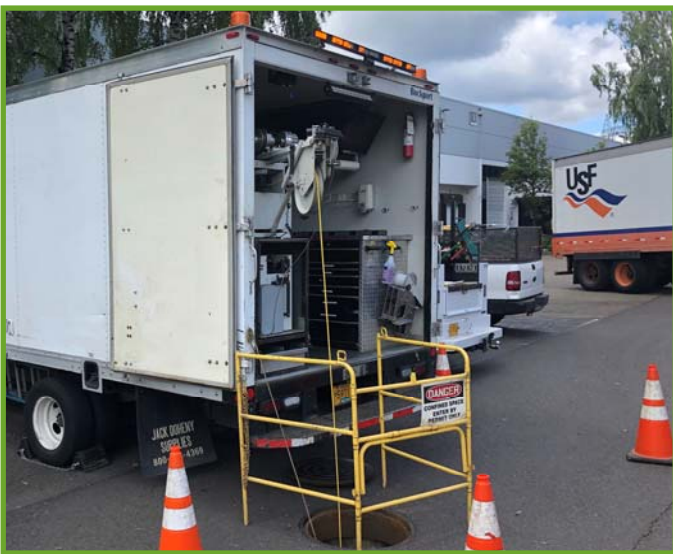
Close Circuit Television (CCTV) Truck
