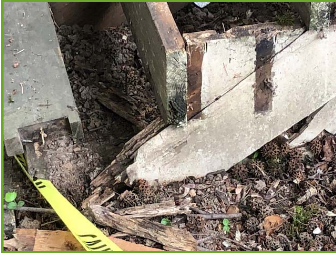
Rotted out stair support
