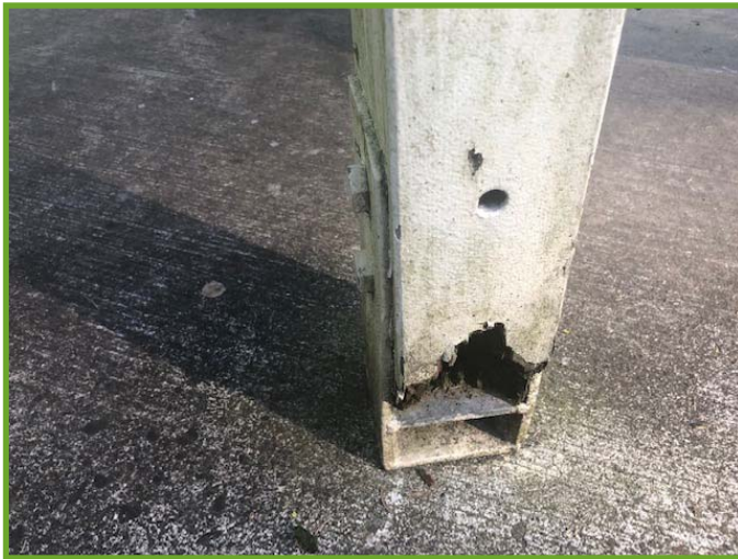
Rotted out supports on Gazebo
