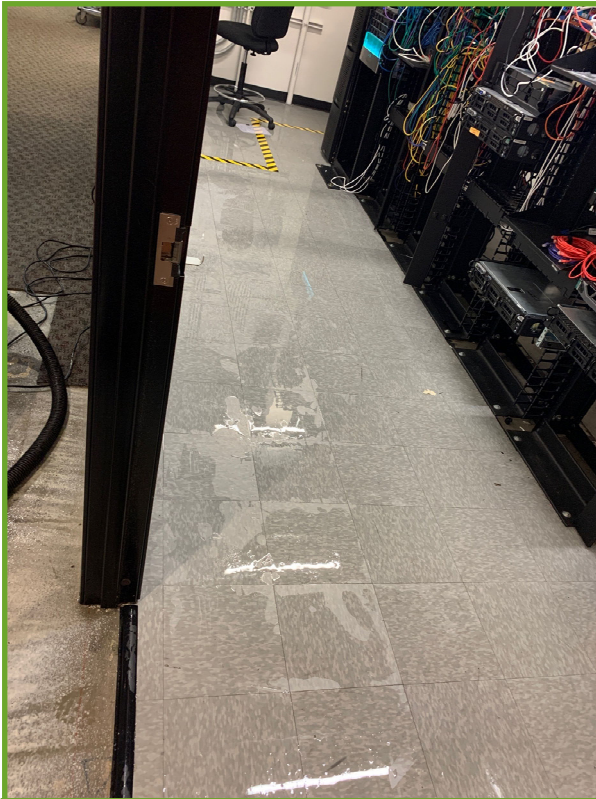
Computer server room— safe but just barely
