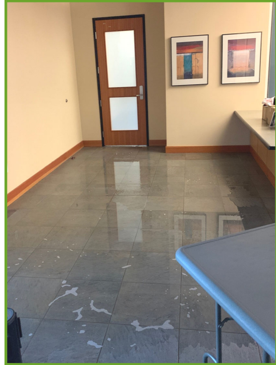
Massive puddle at the front desk
