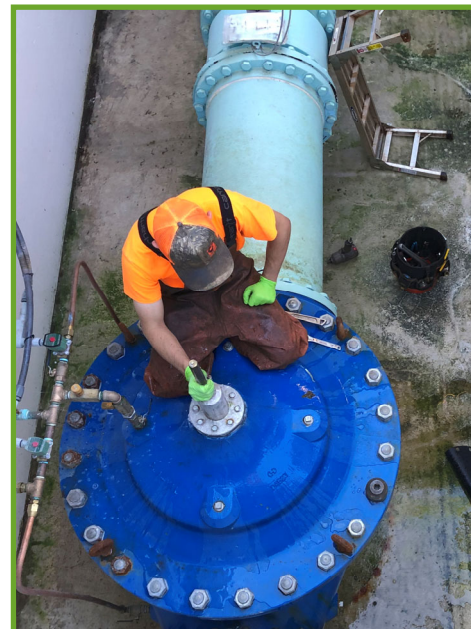
Control valve maintenance
