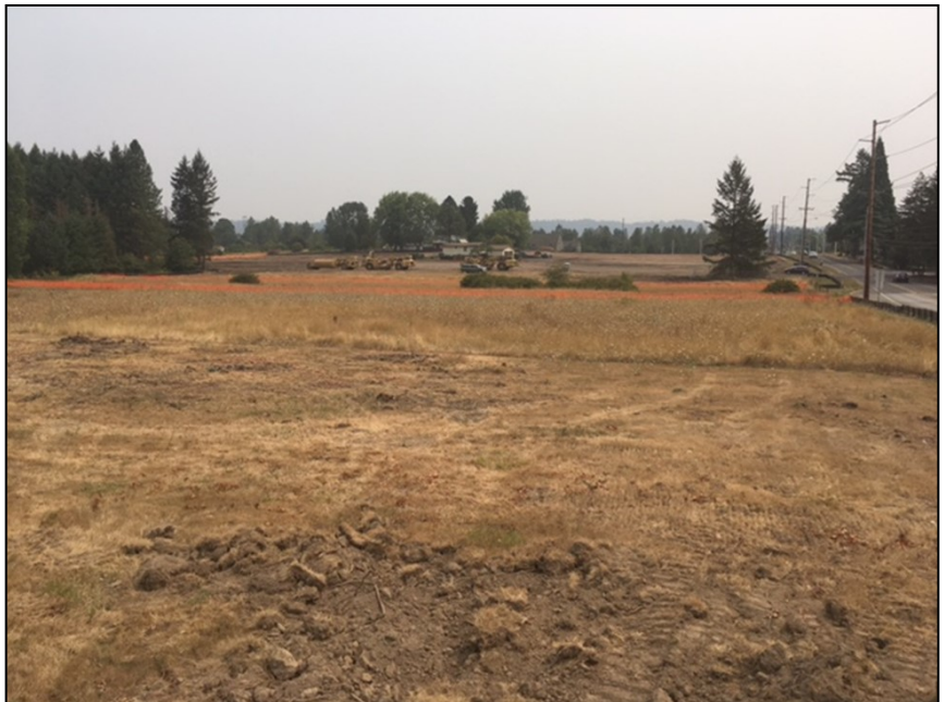
Stafford Meadows—Site Grading is underway. Demolition of three homes and tree removal completed.
