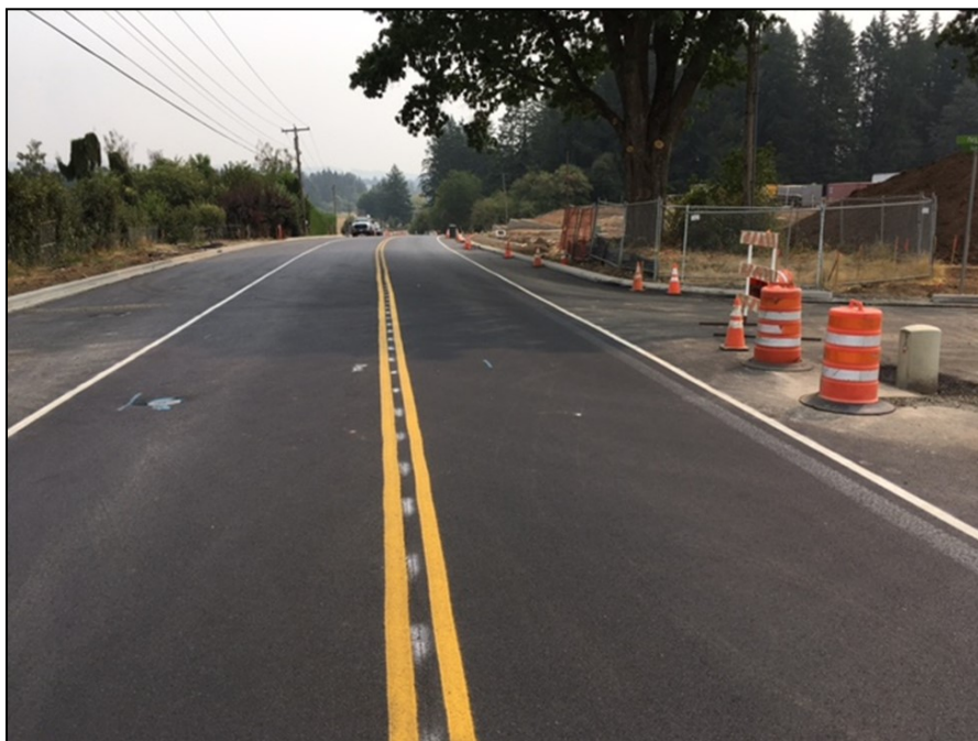
Tooze Road—View east from the new intersection with Paris Avenue. Base lift of asphalt and temporary striping completed. Final striping will include a left-turn lane/center median here.
