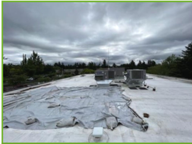
Temporary leak solution: tarp and sandbags
