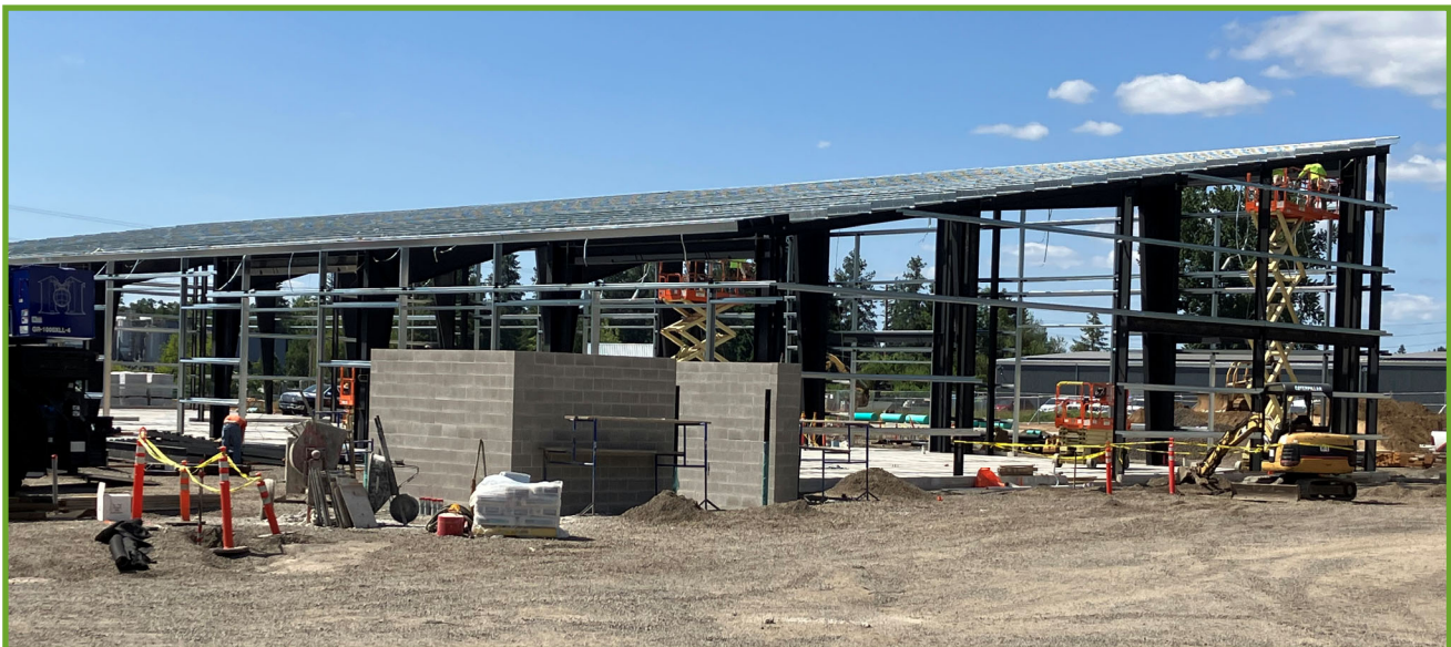
View of the warehouse looking northwest. Block walls for trash enclosure are in the foreground
