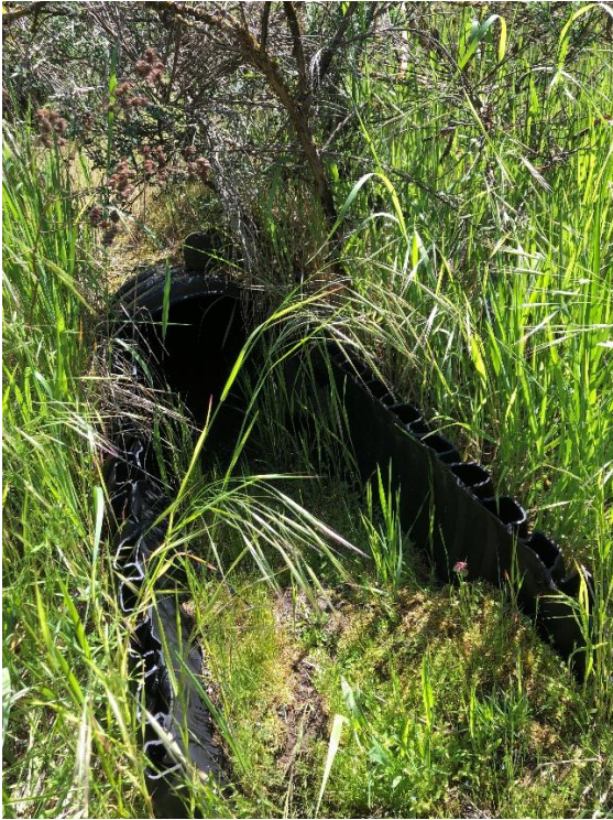
Garden Acres Pond Existing Inflow Pipe (May 2023)
