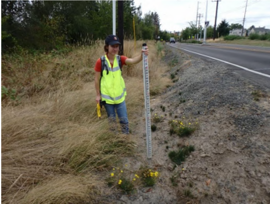
Figure 5. East ditch with sloughing from right bank 2.5 ft height and bottom 2.75 ft width. (node 7)
