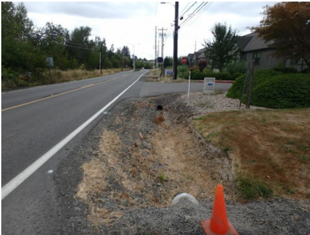
Figure 10. West ditch at church property with gravel and less vegetation, 2 ft depth, 2 ft bottom width and 2:1 side slopes, upstream of driveway crossing (Node 27).
