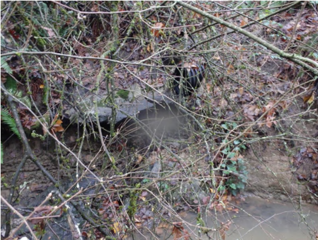
Photo 16 Perched Culvert on Right Bank
