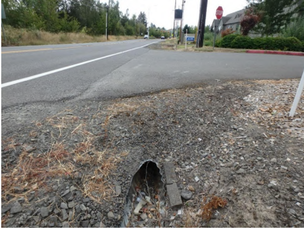
Figure 11. Pipe under church driveway is 10 inch corrugated metal at upstream end and 8 inch plastic at downstream end (Node 27).
