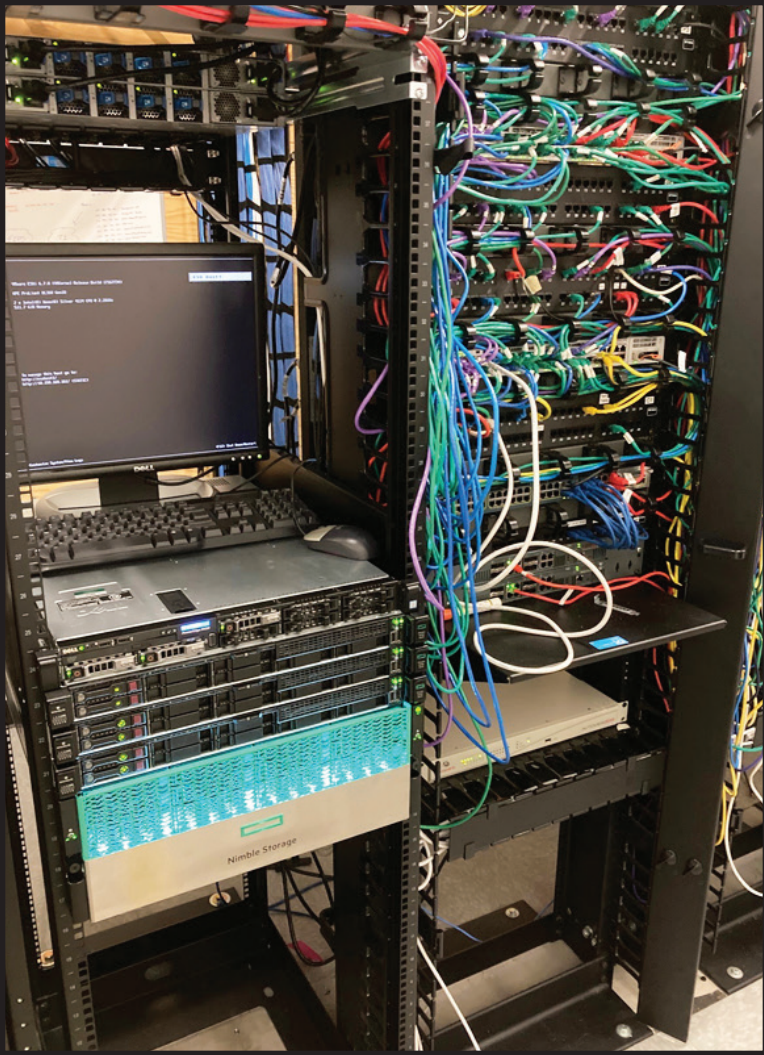
Network racks at City Hall.
