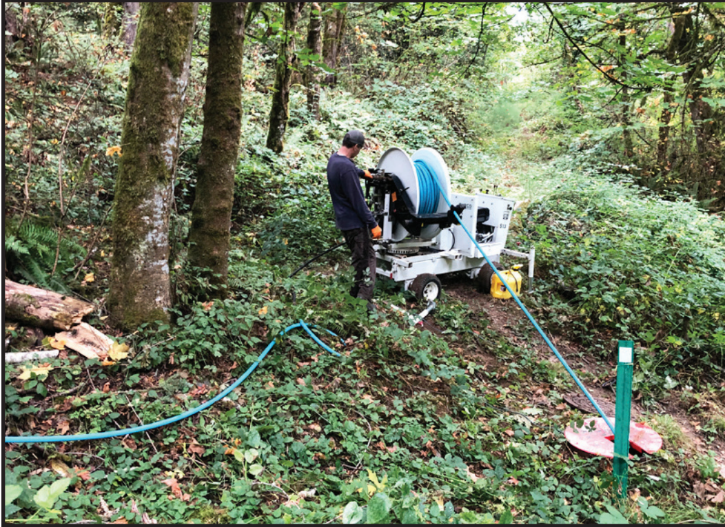
Easement machine being used to clean sewer main lines in difficult to access areas.
