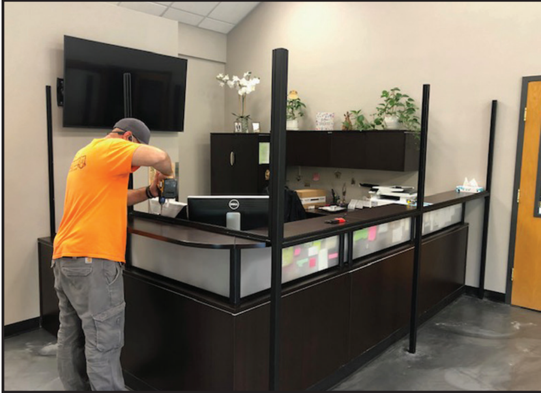
Facilities staff installing custom frames to hold polycarbonate sheets for protection during COVID-19 pandemic.
