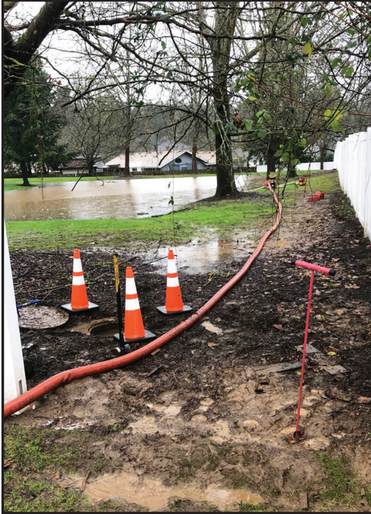
On December 20, 2020, Stormwater staff responded to one of three after-hours floodings.
