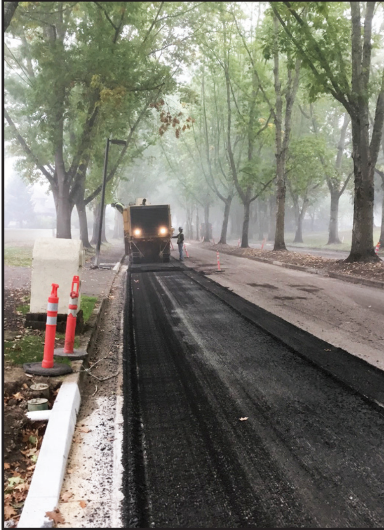
French Prairie Road street grinding prior to paving during Oregon 2020 wild fires.
