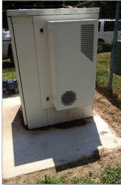
Figure 21: Fiber Distribution Cabinet
