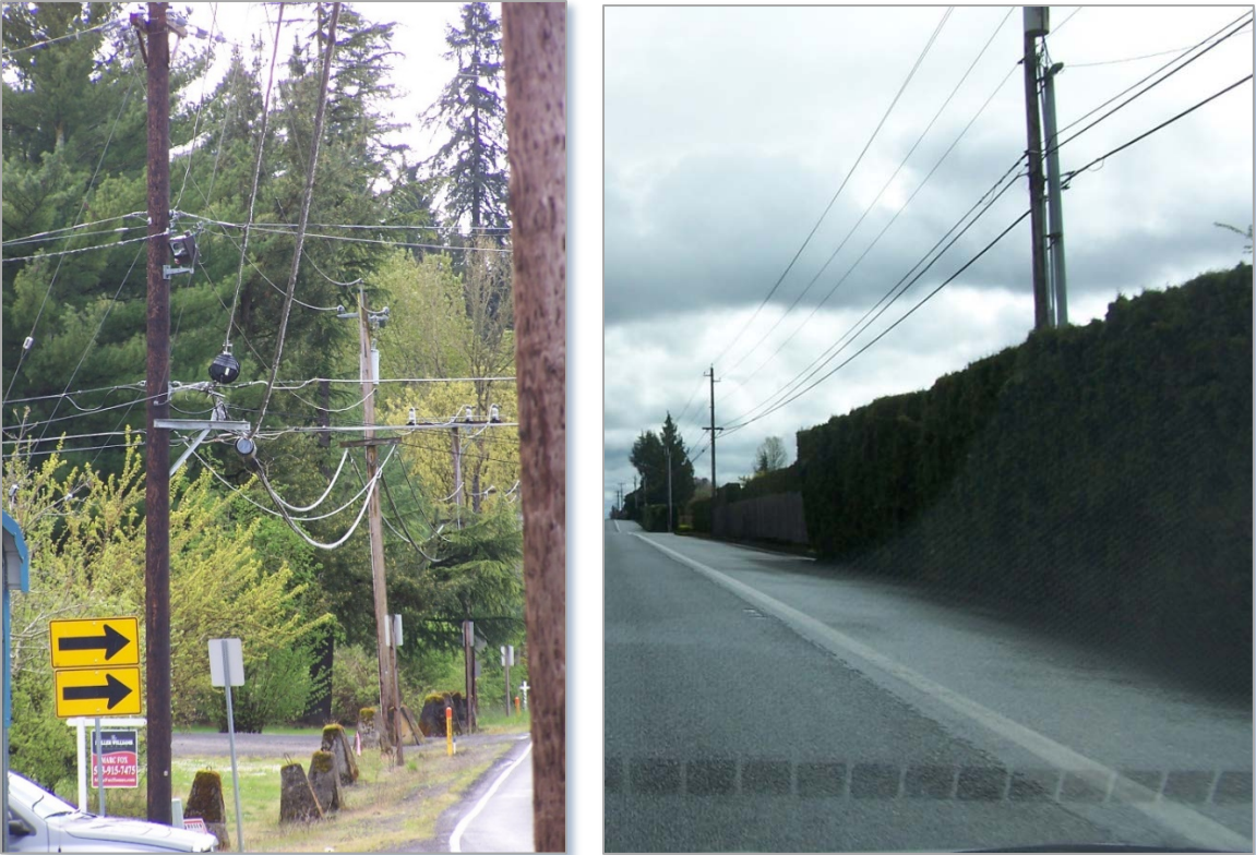
Figure 16: Pole Line to Charbonneau Area
