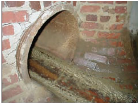
Bacterial growth at this outfall indicates nutrient enrichment and a likely sewage source.
