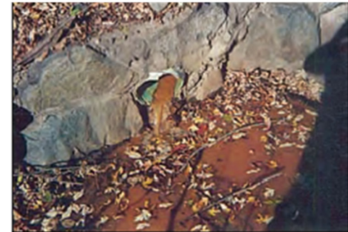
Highly Turbid Discharge Color: Brown; Severity: 3 Turbidity Severity: 3
