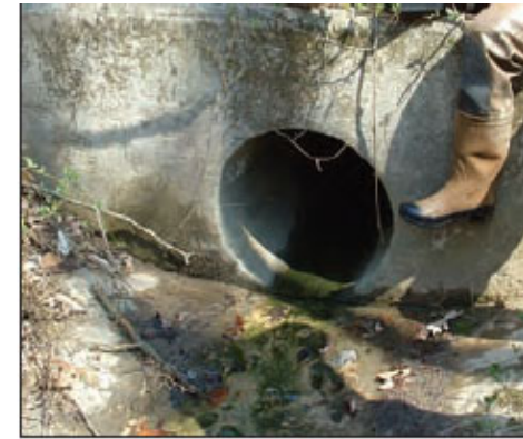
The drainage to this outfall most likely has a high nutrient concentration. The cause may be an illicit discharge, but may be excessive use of lawn chemicals.
