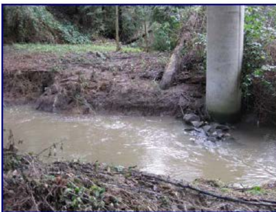
Bank erosion near Wilsonville Road piling
