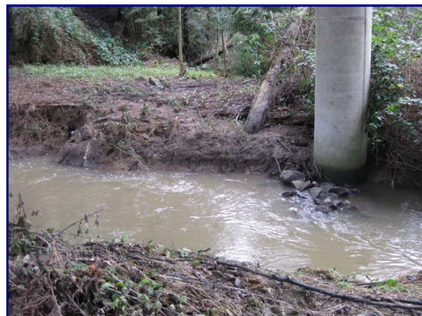
Bank erosion near Wilsonville Road piling
