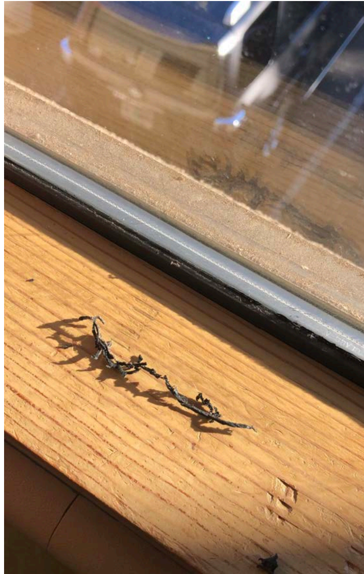
Asbestos containing window caulk
