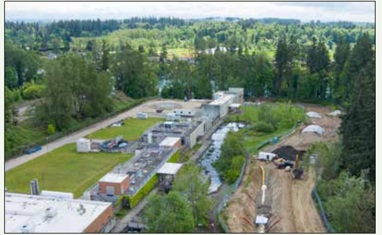
Installing water pipeline at the Willamette River Water Treatment Plant is requiring the temporary closure of the adjacent park this summer.
