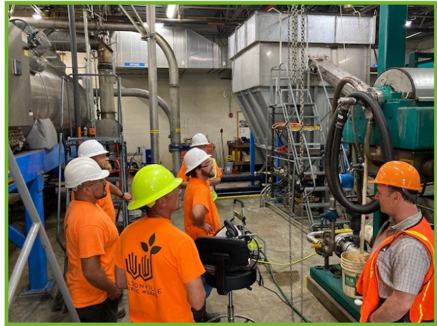
Inside the wastewater treatment plant
