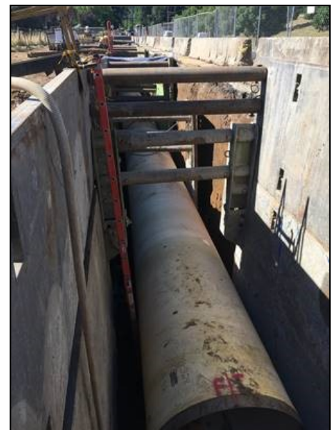
Pipeline under the roadway on Grahams Ferry Rd.
