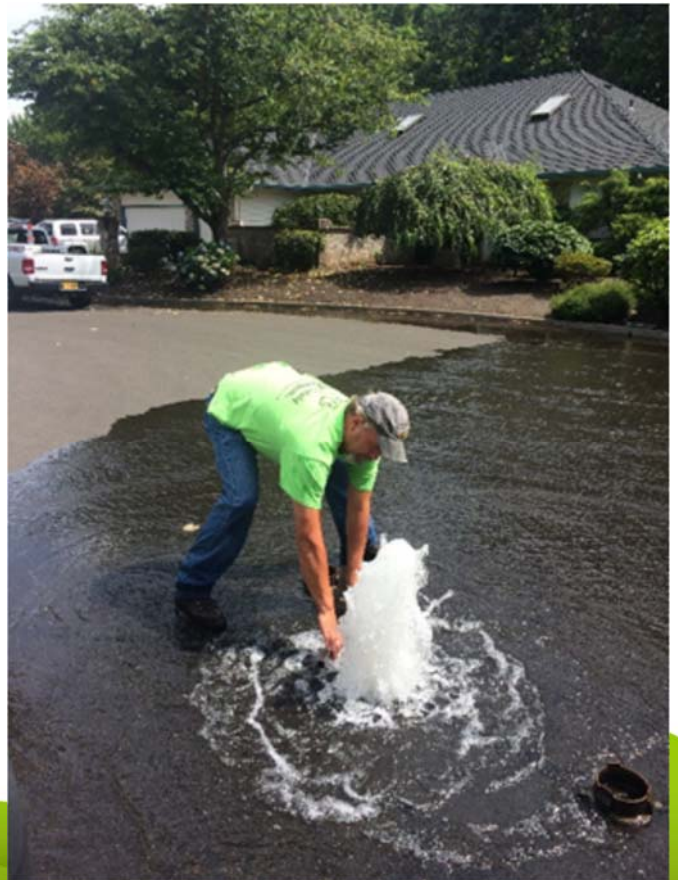
Water Technician Chris Reece opens a blow off valve on Ironwood Court in Charbonneau.
