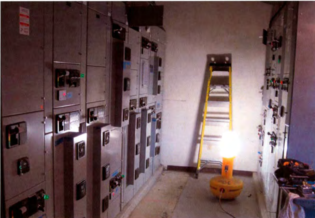
4- Motor control centers.
