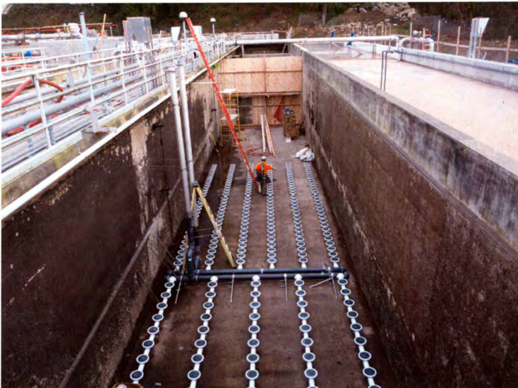
12- Aeration Basin No. 2 air diffusers.
