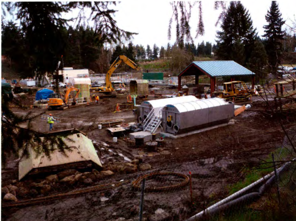
8- Final effluent filters.
