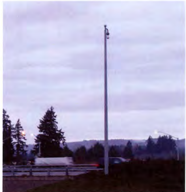
The CCTV camera mounted above the I-5/Wilsonville Road interchange provides a real-time video feed that allows ODOT to monitor and collect traffic information. The video feed is also available to all transportation users on ODOT's Trip Check website.
