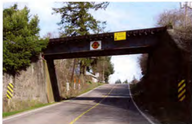
The railroad bridge over Grahams Ferry Road has limited horizontal and vertical clearance. This creates a safety hazard, particularly for bicyclists, pedestrians, and freight traffic.
