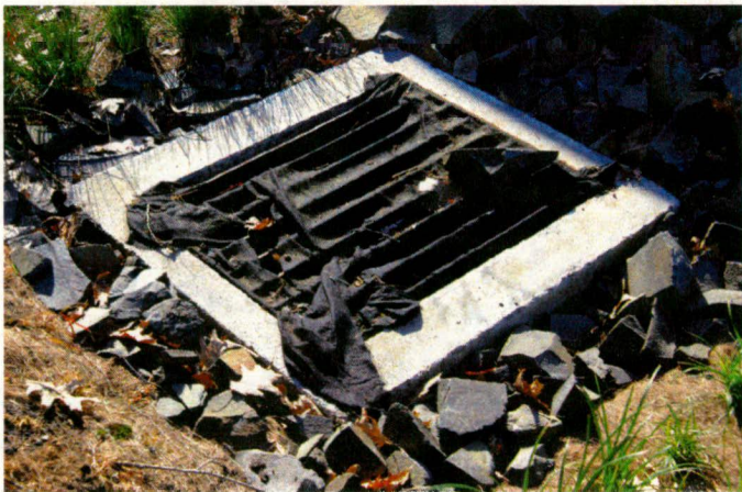
Filter fabric should be removed from outlet
