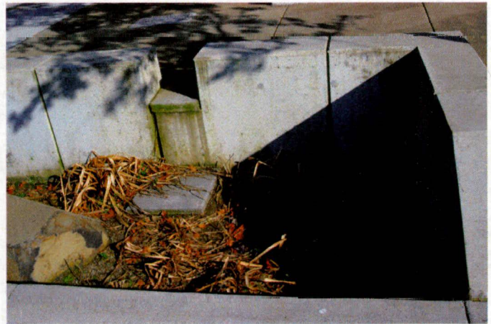
Dead plants need to be replaced
