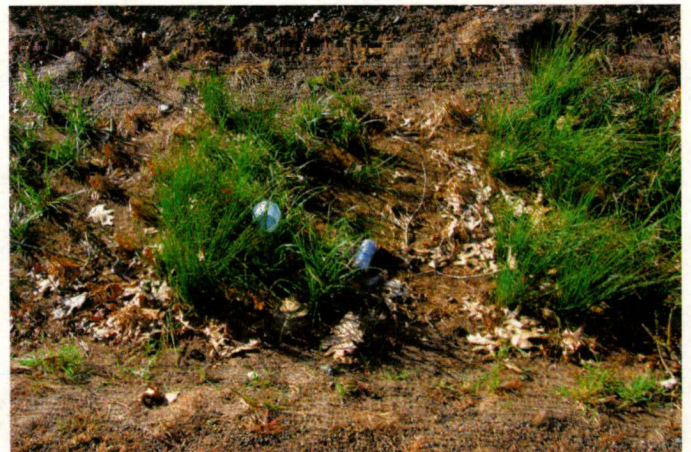
Trash should be removed from swale
