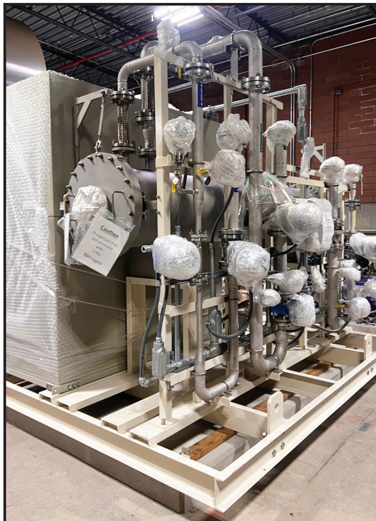
New ozone generator installation underway to expand capacity of the Willamette River Water Treatment Plant (CIP #1144).
