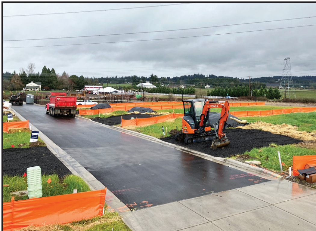
Frog Pond West erosion control.
