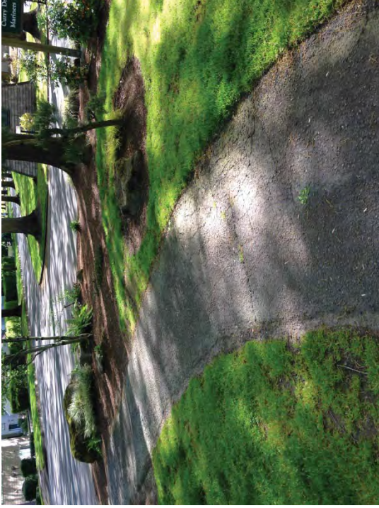
Location #11 – Alligatored asphalt causing trip hazard. Regrade and repave damaged asphalt.
