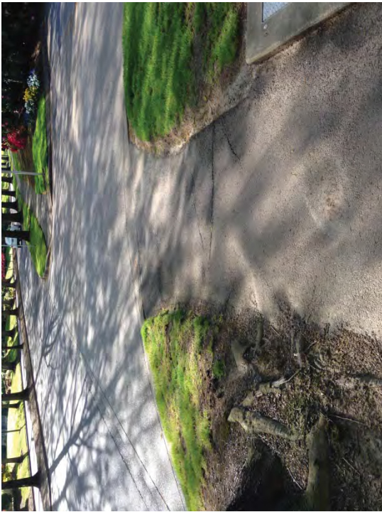
Location #1 – Tree root damage causing tripping hazard. Trim roots where feasible. Install new concrete ADA ramp.
