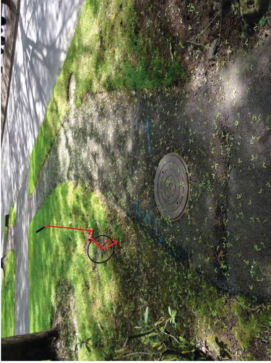
Location #15 – Poor transition to manhole lid causing trip hazard. Regrade and repave asphalt transition.
