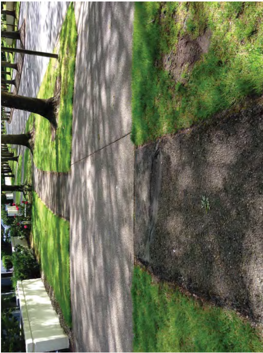
Location #14 – Poor transition to concrete driveway approach causing trip hazard. Regrade and repave asphalt transition.
