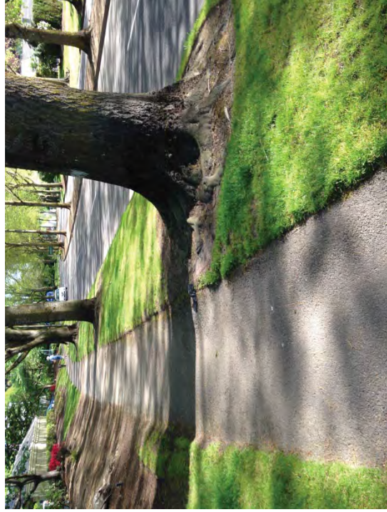
Location #4 – Tree root damage causing tripping hazard. Trim roots where feasible. Regrade and repave lifted asphalt.
