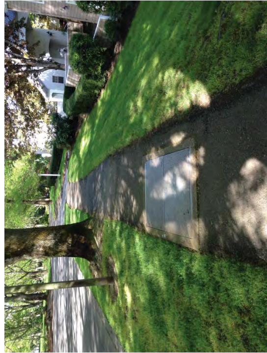
Location #12 – Vault exposure and tree root damage causing trip hazard. Trim roots. Regrade and repave damaged asphalt.
