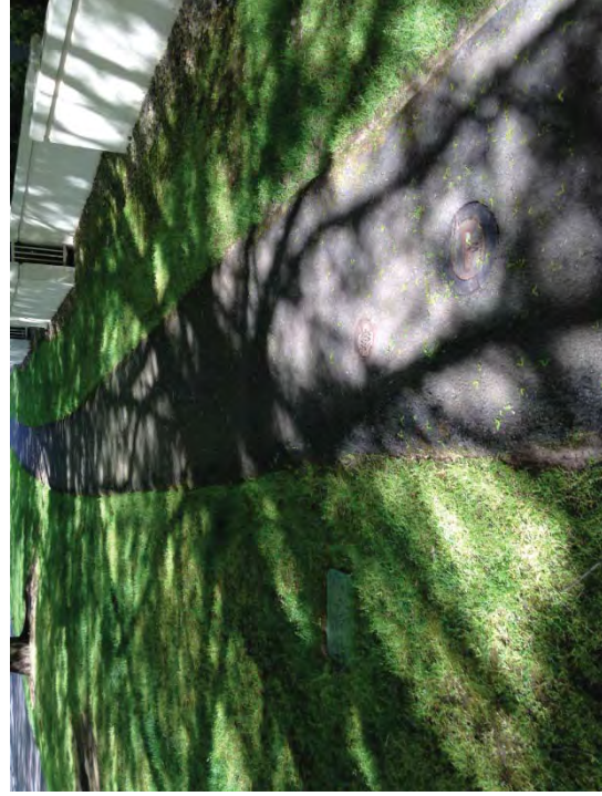
Location #13 – Valve boxes causing trip hazard. Regrade and repave damaged asphalt.
