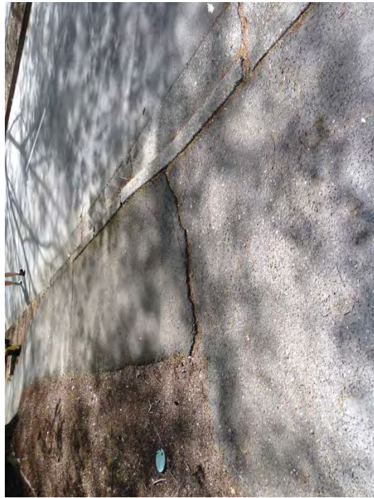
Location #16 – Poor transition to driveway approach causing trip hazard. Regrade and repave asphalt transition.
