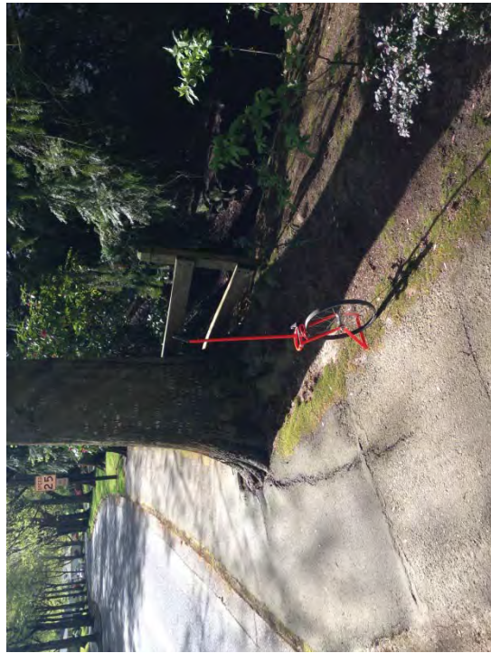
Location #3 – Tree root damage causing tripping hazard. Remove tree, regrade and repave lifted asphalt.
