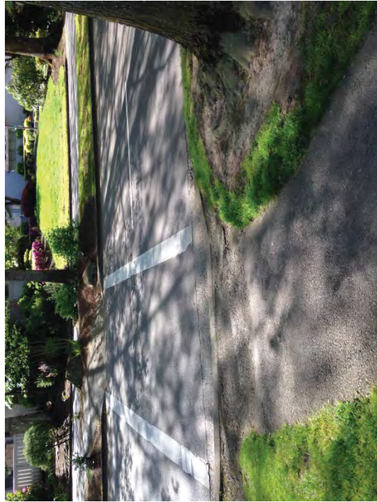
Location #7 – Tree root damage causing trip hazard. Trim roots where feasible. Install concrete ADA ramp.
