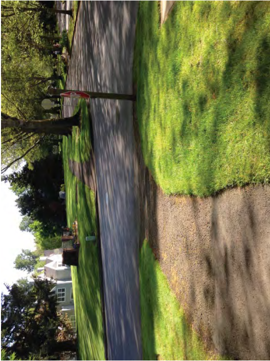
Location #5 – Surface consists of loose rock asphalt and is slippery. Install concrete ADA ramp and regrade and transition with asphalt.
