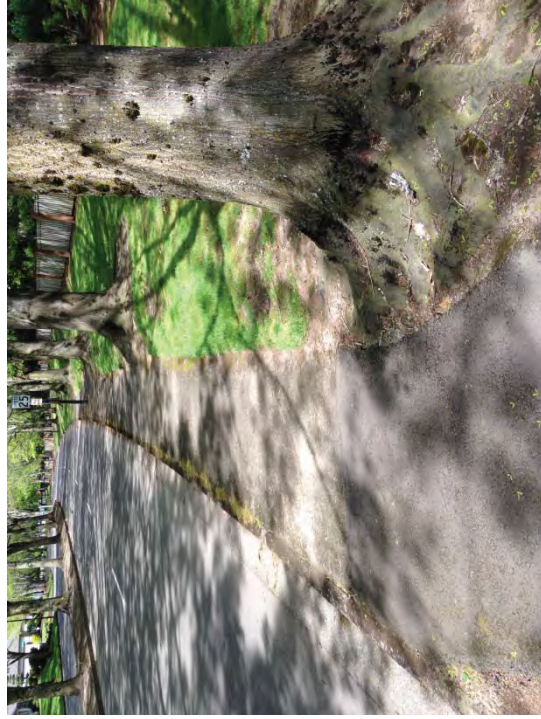
Location #17 – Tree root damage causing trip hazard at three locations. Trim roots where feasible. Regrade and repave lifted asphalt.
