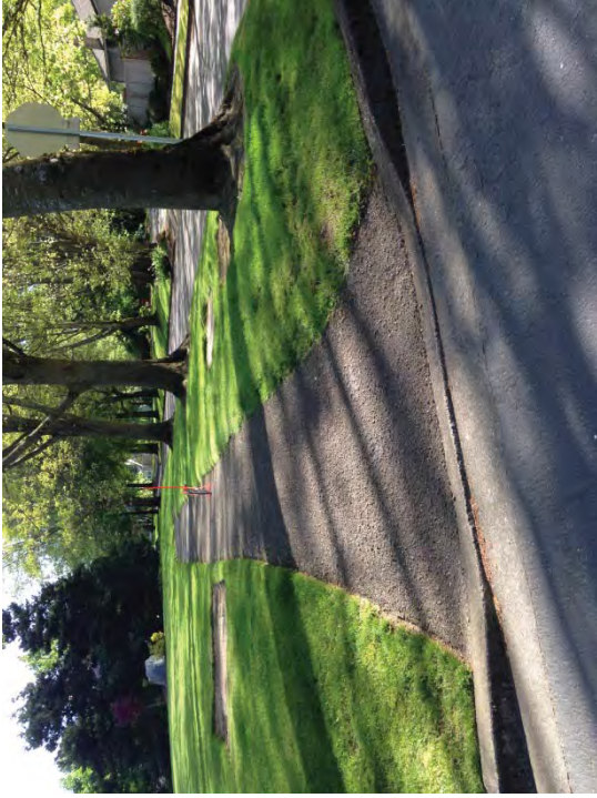
Location #6 – Surface consists of loose rock asphalt and is slippery. Install concrete ADA ramp and regrade and transition with asphalt.
