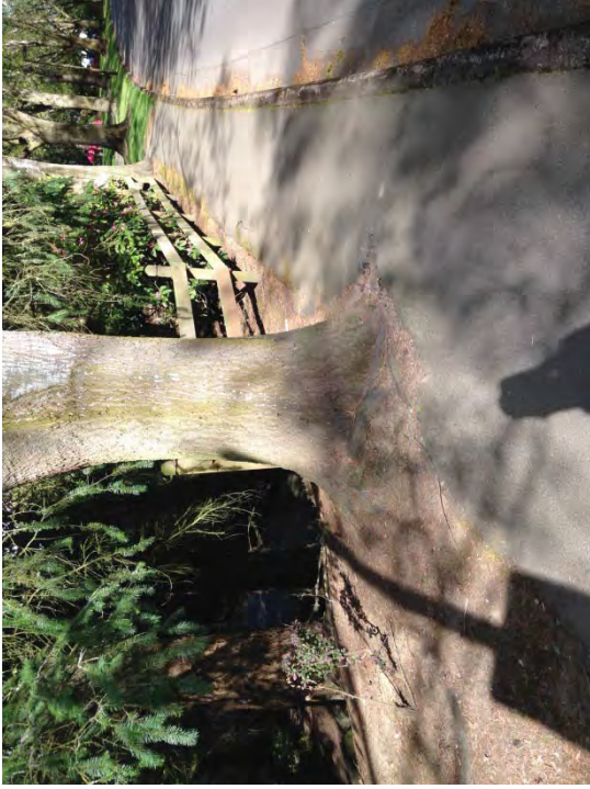
Location #2 – Tree root damage causing tripping hazard & narrow passage. Remove tree, regrade and repave lifted asphalt.
