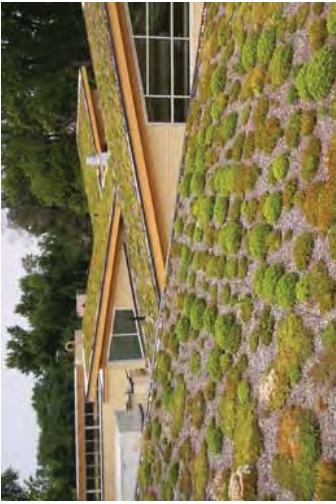
Green Roof (Reduces roof runoff and improves building insulation)
